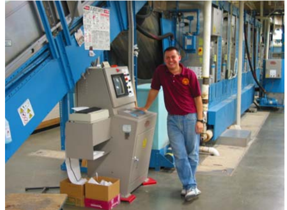
Tunnel Washer System
